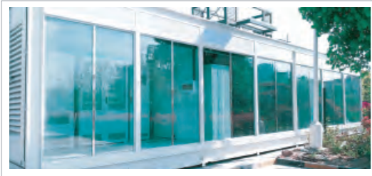
SAIC-GM-Wuling 1MWh Step-Utilization ESS Project
