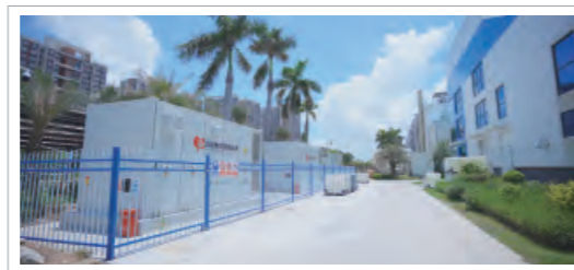
Zuhai Great Power Production 29.77MWh Project
