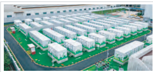
Nanning 100MWh Energy Storage Project
