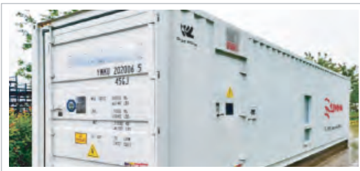
Croatia 17MWh Photovoltaic and Storage Complementary Project
