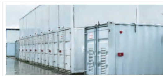
State-Owned Shipyard 100MWh Energy Storage Station Project
