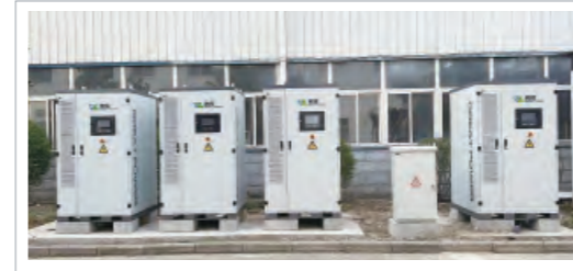
Zhumadian Zhongji Huajun 2.8MWh Project
