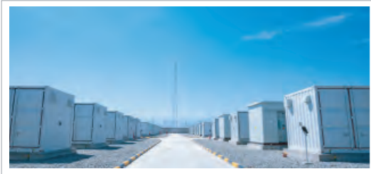
Jimusaer 150MWh Project
