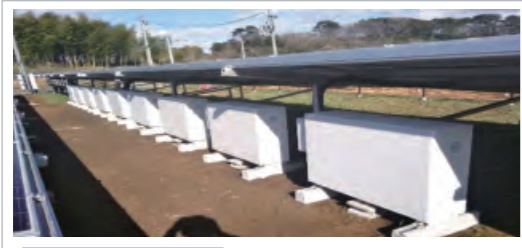
Japanese 0.2GWh Factories, nursing homes, low-voltage power plants and warehouses in Tokyo, Osaka and Kagoshima, Japan
