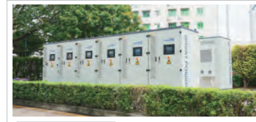
Guangzhou Production 7.33MWh Project
