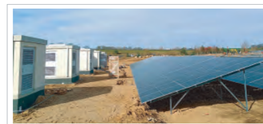
Germany 16.77MWh Containerized Energy Storage Project
