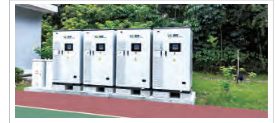
Shenzhen Yinghe 3.26MWh Project
