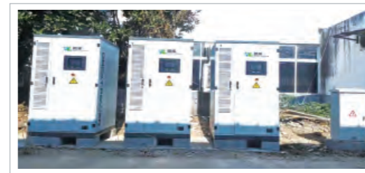
Runan Yuxin 1.5MWh Project
