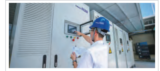
Guangzhou Xinli 2.33MWh Project
