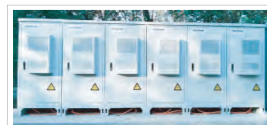
India 2MWh High-Grid Photovoltaic Storage Project
