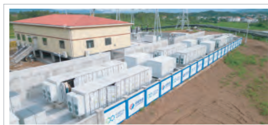
Ji'an 15MWh Agro-Photovoltaic Complementary Project
